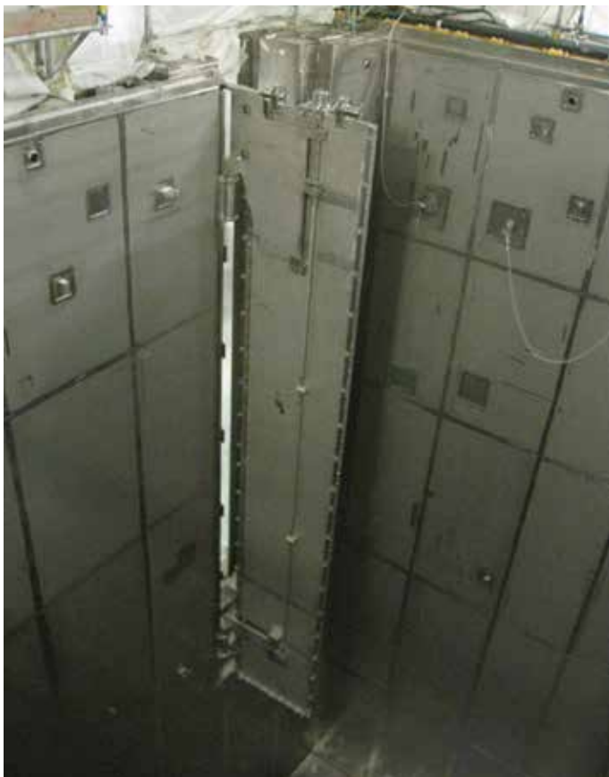
Olkiluoto 3: Pool Liner with Gate
