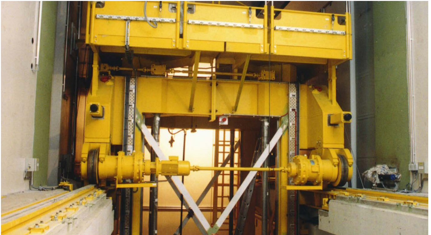
PKA Gorleben; Spent Fuel Cask Transfer Machine
