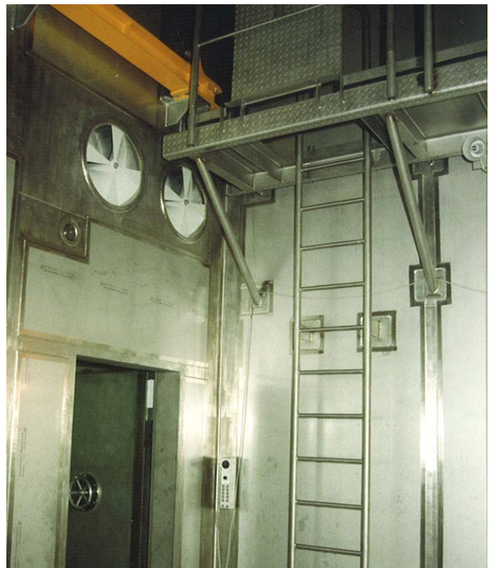
Ventilation Screw with Penetration in Hot Cell Wall
