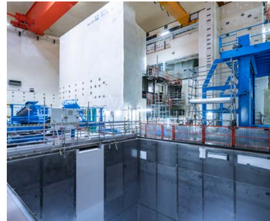
The two wire saws in front of the fuel element storage pool
